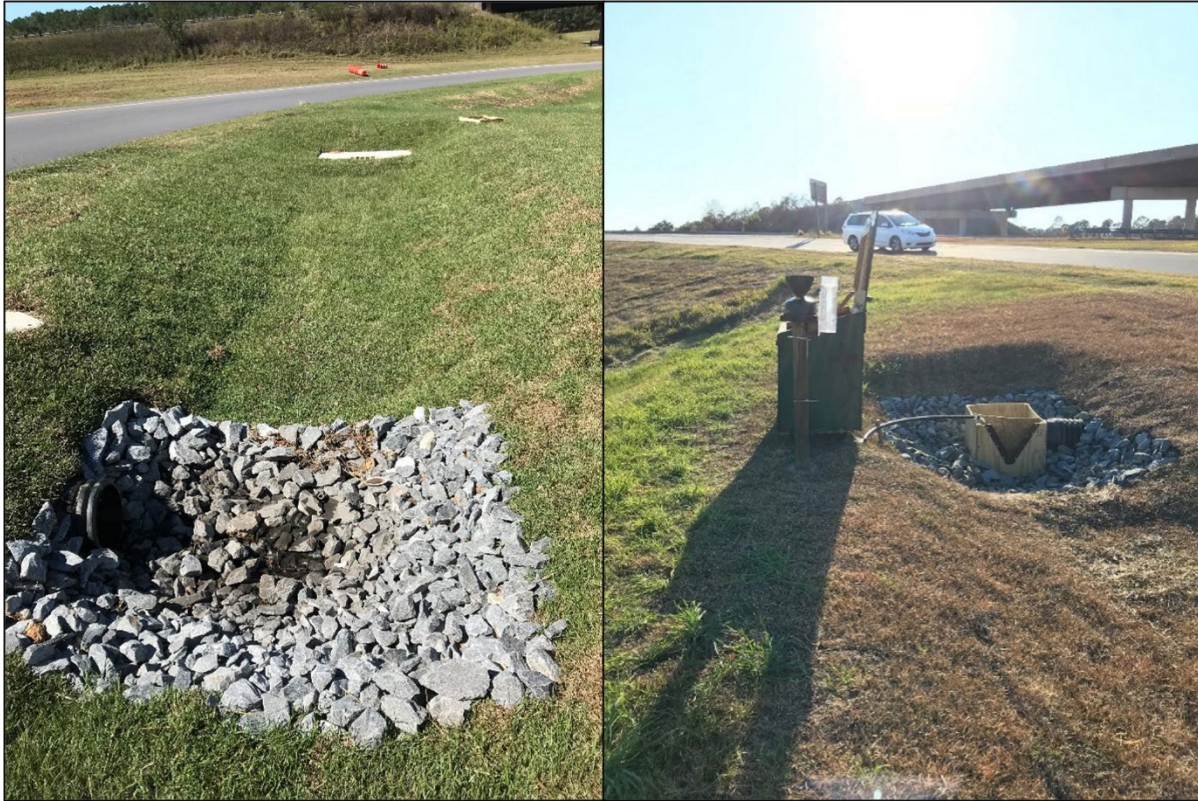
Figure 14. Inlet and forebay (left) and weir box (right) for BSN and BSS bioswales
